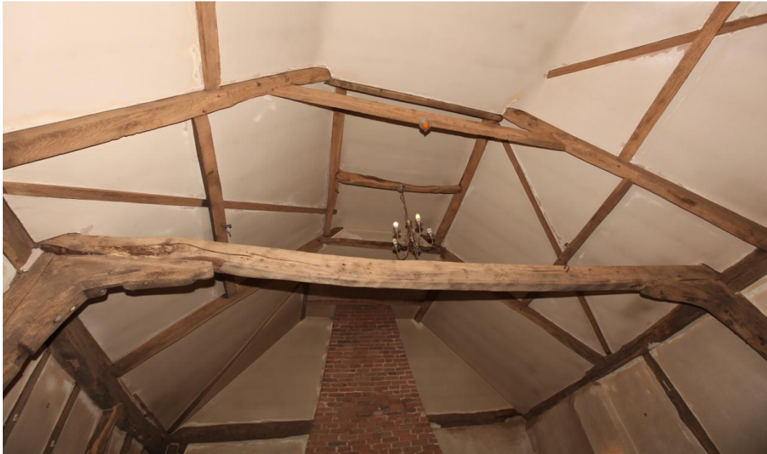
Illus. 8. The late-18 th century rebuilt roof of the Tudor hall, seen from the south. The tie-beam spanning the walls is also a replacement, along with its bolted knee-braces. The original tie-beam was arch-braced like its counterpart on the south (illus. 6), as indicated by mortises in the original wall posts.
