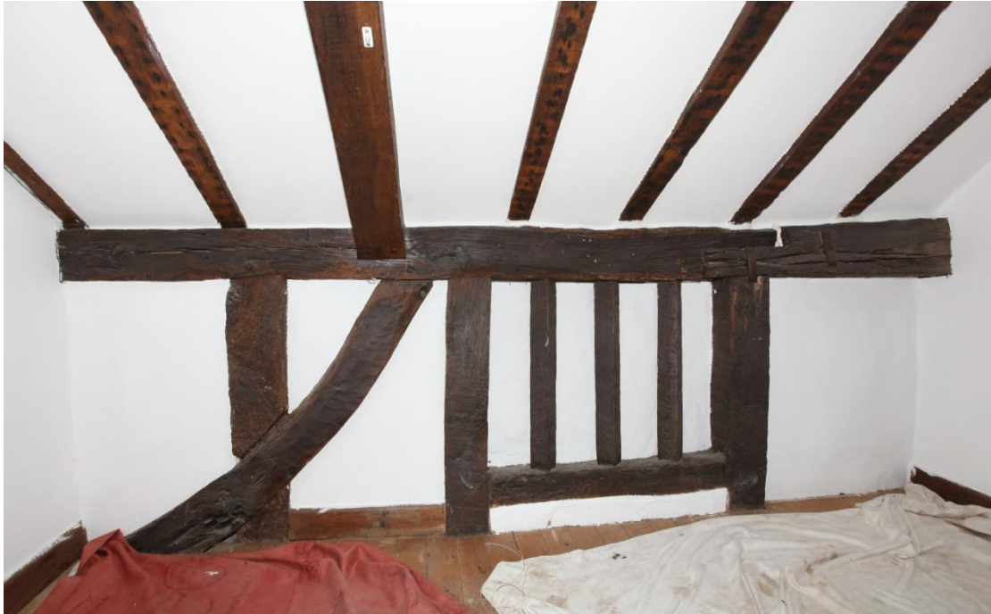
Illus. 10. The original diamond-mullioned 16 th century window in the back wall of the first-floor room above the bar area shown in illus. 9 above (A1, i.e. the original service chamber). The curved wall brace is also original, as is the ‘edge-halved and bridled’ scarf joint in the roof-plate to the right. Joints of this kind were standard in the 16 th century but were quickly superseded after circa 1600.
