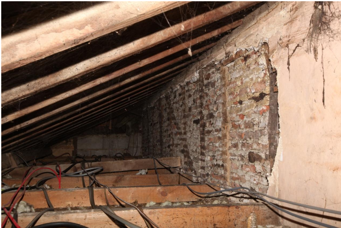
Illus. 15. The original northern external wall of the 18 th century wing (B), now exposed in the lean-to roof above the modern kitchen (the exterior of the wall shown in illus. 14 above). The studwork and diagonal primary bracing is typical of the 18 th century, as is the infill of re-used brick as opposed to the wattle-and-daub used in the Tudor house (A).
