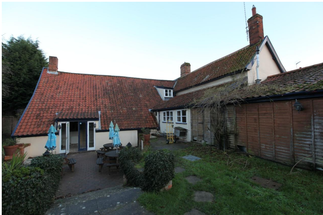
Illus. 4. The rear of the inn, showing the unglazed pantiles of the 16 th century structure (A) and its lean-to extension on the left and the formerly open-sided lean-to kitchen and adjoining sheds on the right. The roof of the lean-to kitchen has protected the original external pargeting and 19 th century ‘Suffolk Pink’ of the 18 th century wing (B), as shown in illus. 15 & 16 below).
