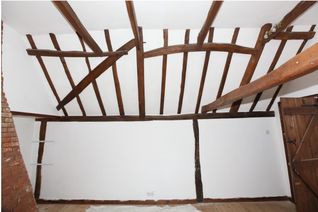
Illus. 16. The typical 18 th century roof structure of staggered butt-purlins in the northern internal wall of the rear wing (above rooms B3 to the left and B2 to the right).
