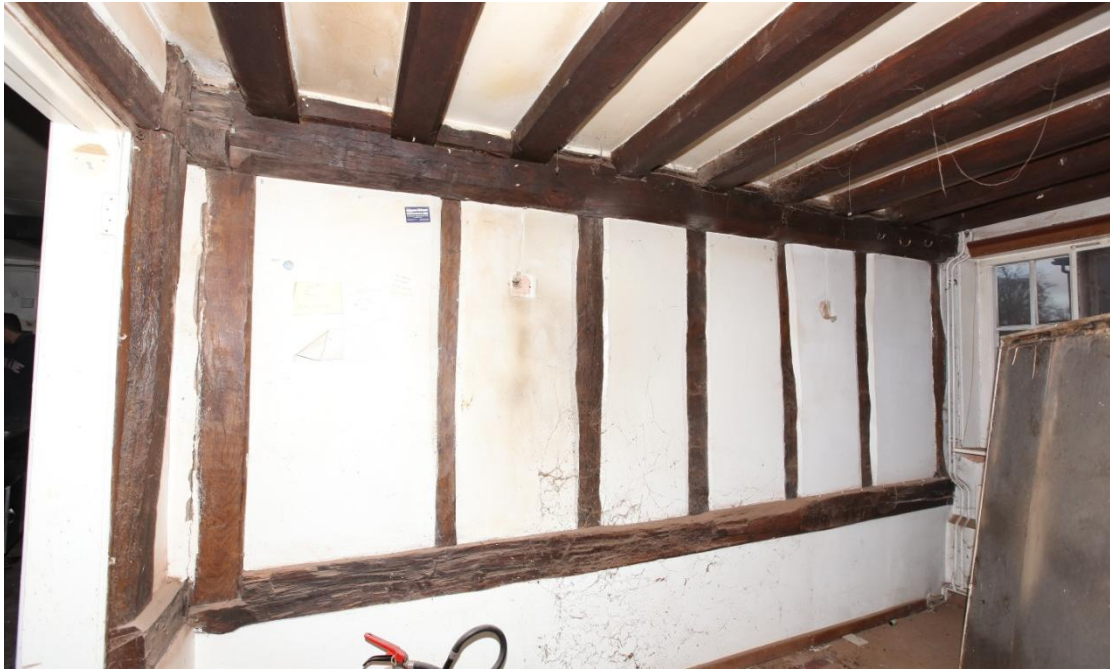
Illus. 14. The rear kitchen of the 18 th century wing (B3) viewed from the west, showing the original solid partition adjoining the central room (B2). This room contains a complete, high-quality 16 th century ceiling with neatly chamfered and step-stopped joists which extends into the central room. The common joists are tenoned to the contemporary principal joist, which is chamfered and stopped at both ends, but the vertical studs are nailed additions. Remarkably, there is no evidence of intact 16 th century fabric in the external walls, and the entire ceiling appears to have been re-used from an older building of the same width.
