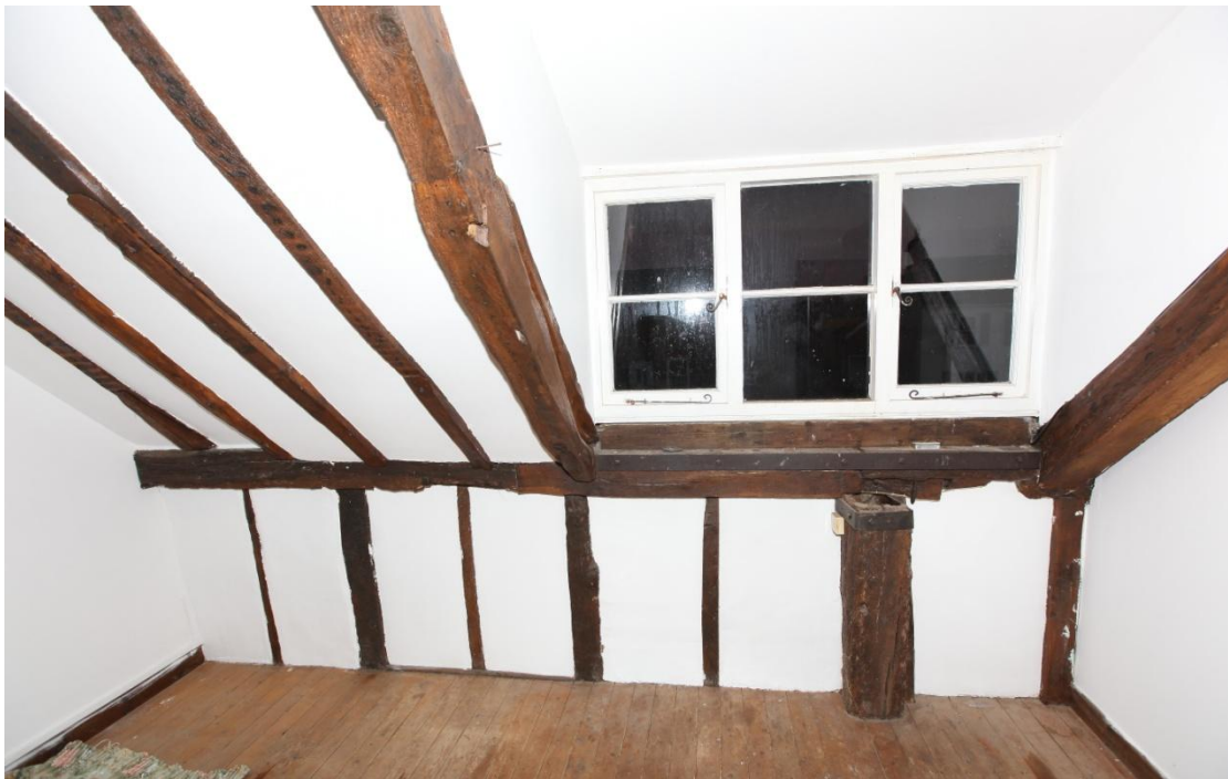
Illus. 11. The dormer window in the front wall of the first-floor room above the barn (A1). The studs here are later replacements, along with the roof timbers, but the large post beneath the window remains in situ and marks the south-eastern corner of the Tudor house. The empty diamond-mullion mortises of an original window can be seen in the underside of the roof-plate on the left. This window would have matched the intact example in the opposite wall shown in illus. 10 above.
