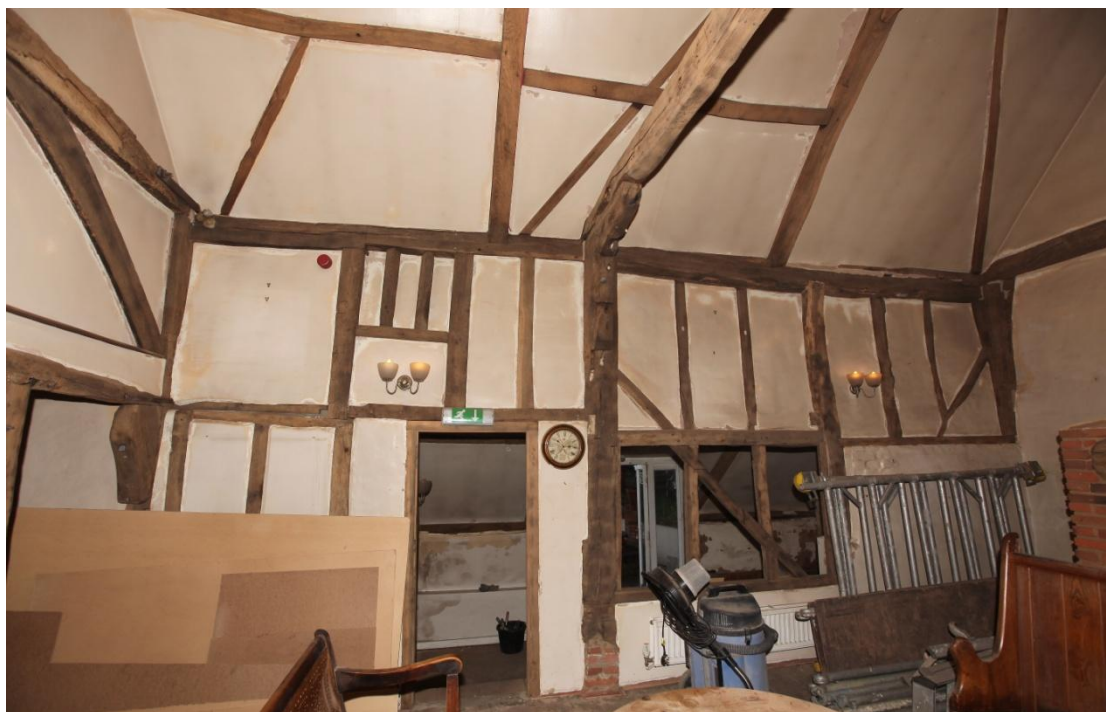
Illus. 5. The rear (western) internal wall of the 16 th century structure (A2). Now open to its late-18 th century roof this room originally contained a ceiling and formed the two-bay hall of the Tudor house. The studs to the right of the central post have been replaced, leaving only the roof-plate in situ , but the diamond mullions of the first-floor window to the left are entirely original. 16 th century windows typically lacked glass, but contained square mullions set diagonally and were closed by internal shutters. The outline of the blocked original back door can be seen to the left of the present door into the lean-to extension.
